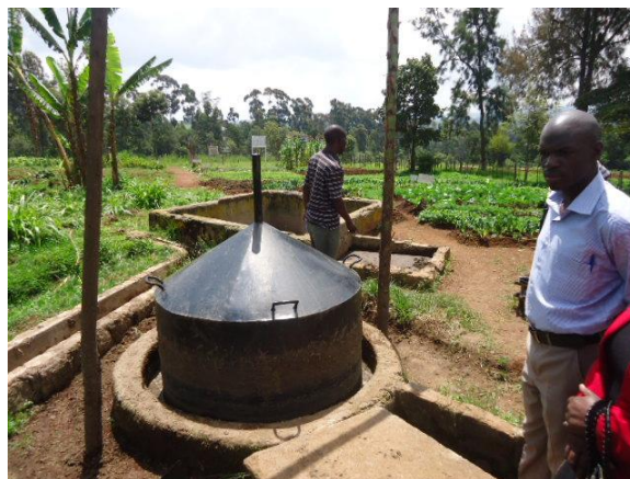
Floating dome biogas generation facility at Baraka Agricultural College.
