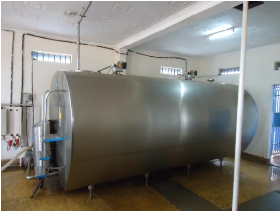
Milk cooling unit at Kabiye Dairies.
